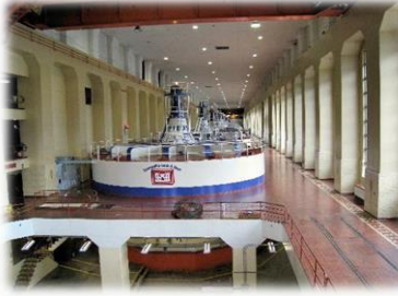
Control Rm Fire Protection
