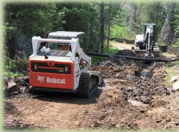
Remote Site Waterline
