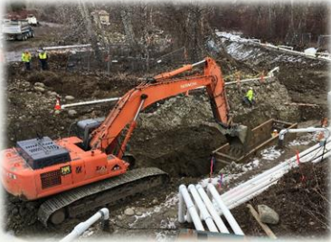
Fish Infiltration Gallery
